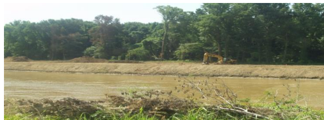
Construction along the bank of the Tallahatchie River Item 6B near Phillip, MS
