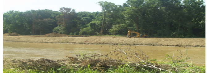
Construction along the bank of the Tallahatchie River Item 6B near Phillip, MS
